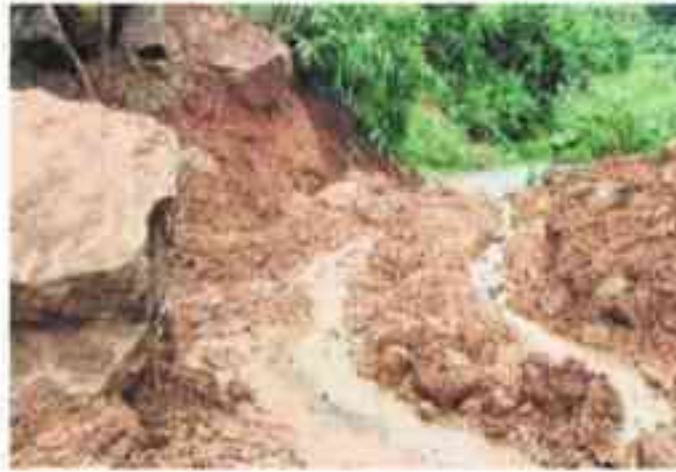
A section of the Shankuda-Khiliganda ghat road after the landslide | careers
