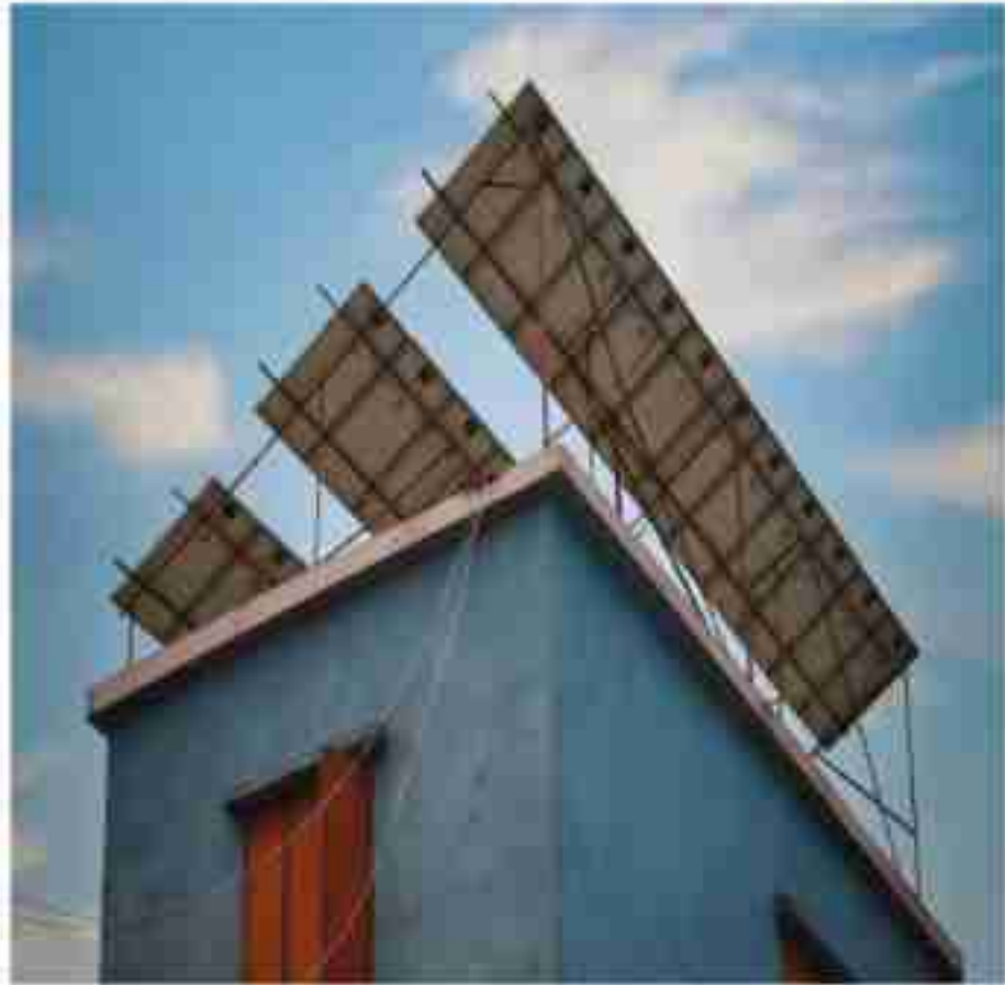
All 200 eligible households in Matikhola village have been equipped with 1 kW rooftop PV systems under the ULA model. Image Credit/Source: Kaitir/ Rishwan/ Nysal/ Pevini
